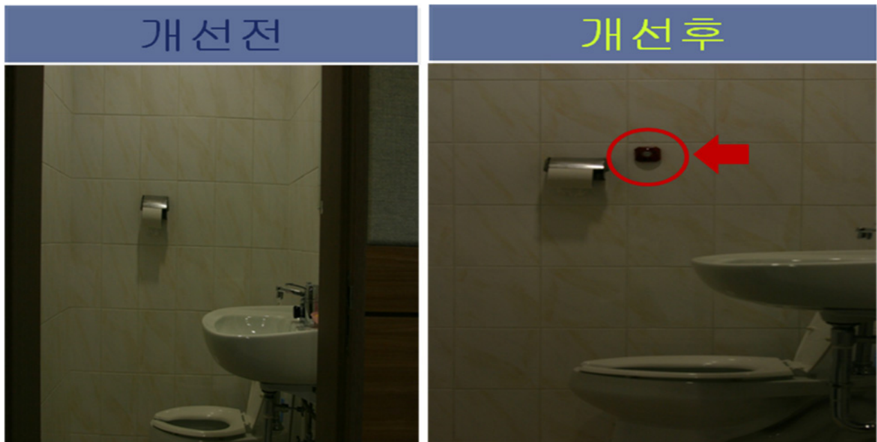
Fig. 14. Bell installed in the bathroom.
